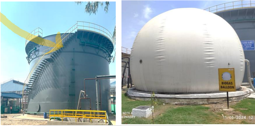
UASBR & Biogas Balloon
